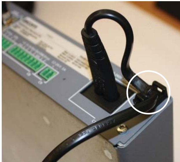
Figure 13. Cable ties on the network cable side
